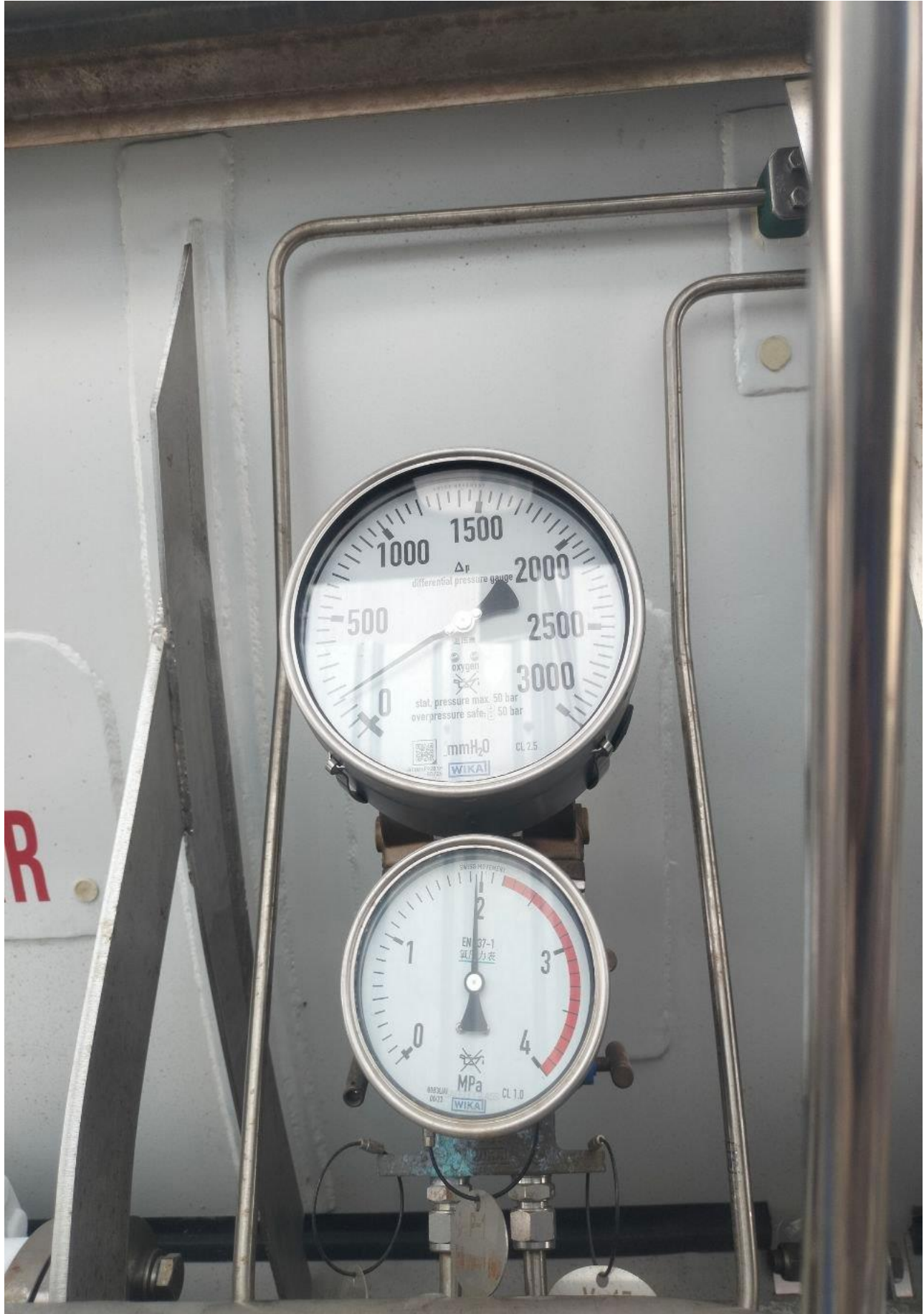
Gauge On Tank
